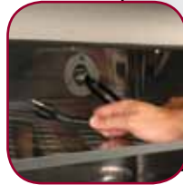
Throughwall Access Port
