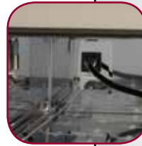
Interior Electrical Outlet
